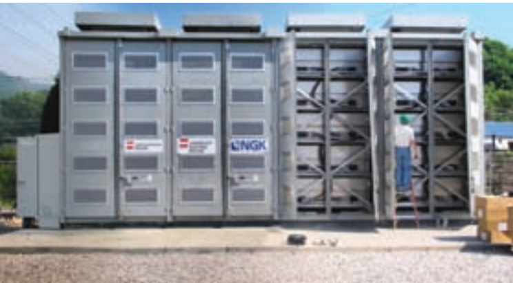
The sodium sulfur battery installation at AEP's Charleston substation is designed to enhance grid reliability.
