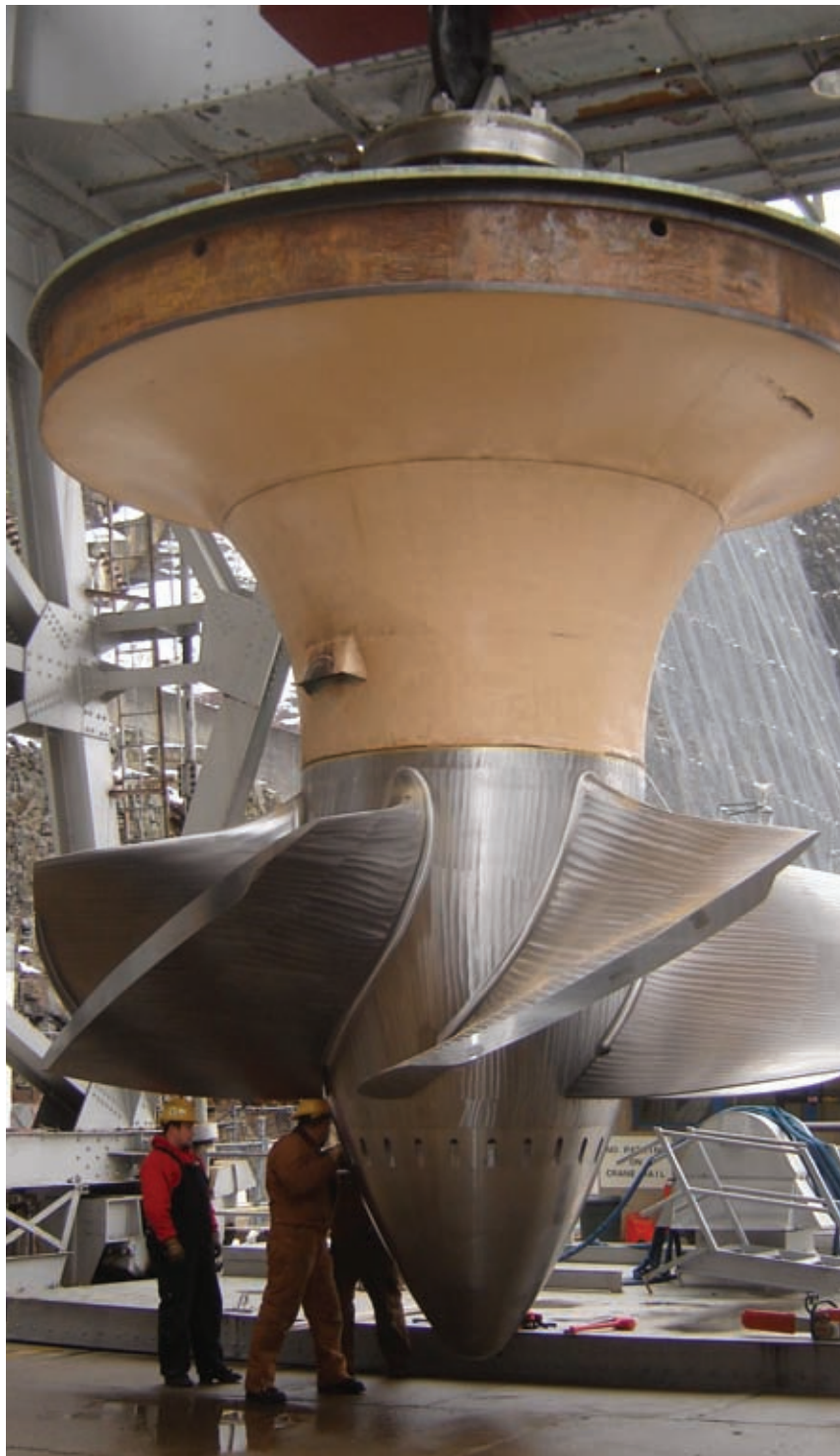
Avista crews perform final inspection of the new, high-efficiency turbine runner and shaft assembly just prior to setting it in place at the Cabinet Gorge Project powerhouse.
