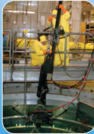
New Core Shroud Inspection Technology
