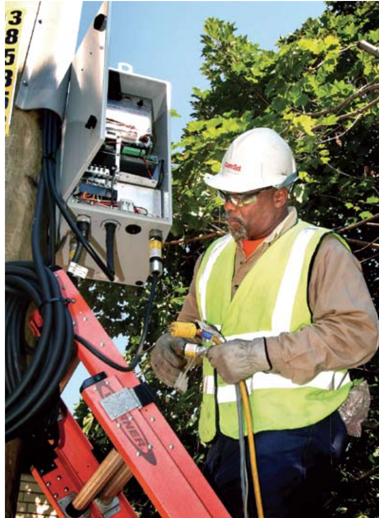
▲ Chuck Brown, a principal technician with ComEd distribution testing, tests the controller cabinet near a recently installed midcircuit reclosure on Chicago's North Side.
